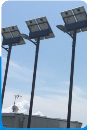
PJU Tenaga Surya (4 m - 12 m)
